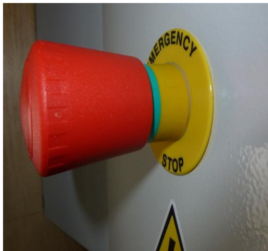
Fig.3 - The emergency stop switch in the on position allowing the compressor to start.
