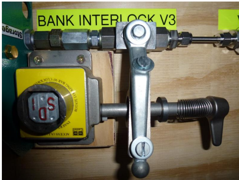
Fig. 9 - The bank interlock system with the bank offline (note the Castell key is removed)
