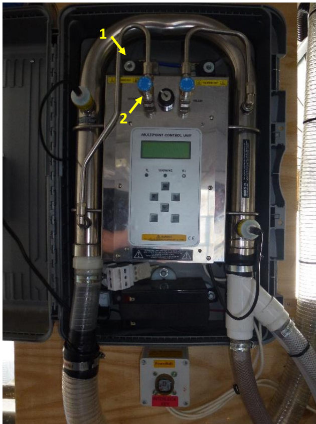
Fig. 7 - The blending panel with the Castell interlock power switch underneath.
