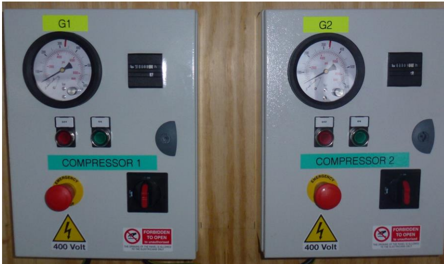
Fig. 2 - The compressor remote control panels.
